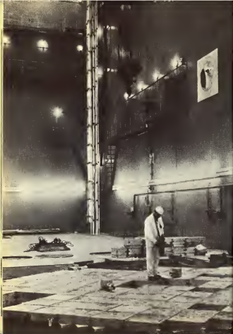
Reactor room at Belyar atomic power station.
